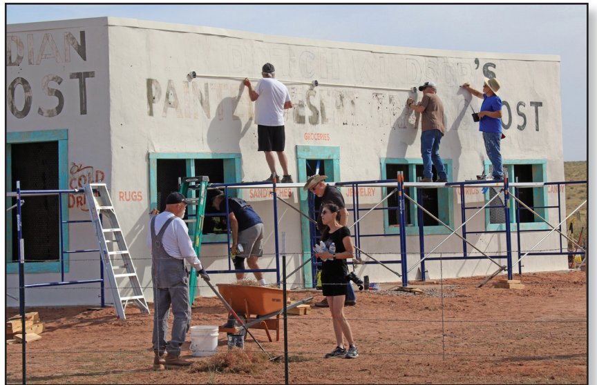
Artist Jerry McClanahan (far right) works on lettering while lighting conduit to match the original is installed.
