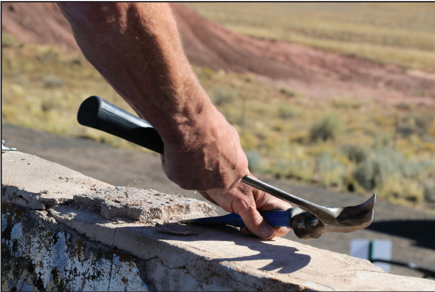
The parapet walls required labor intensive prep for stucco repair and capping.
