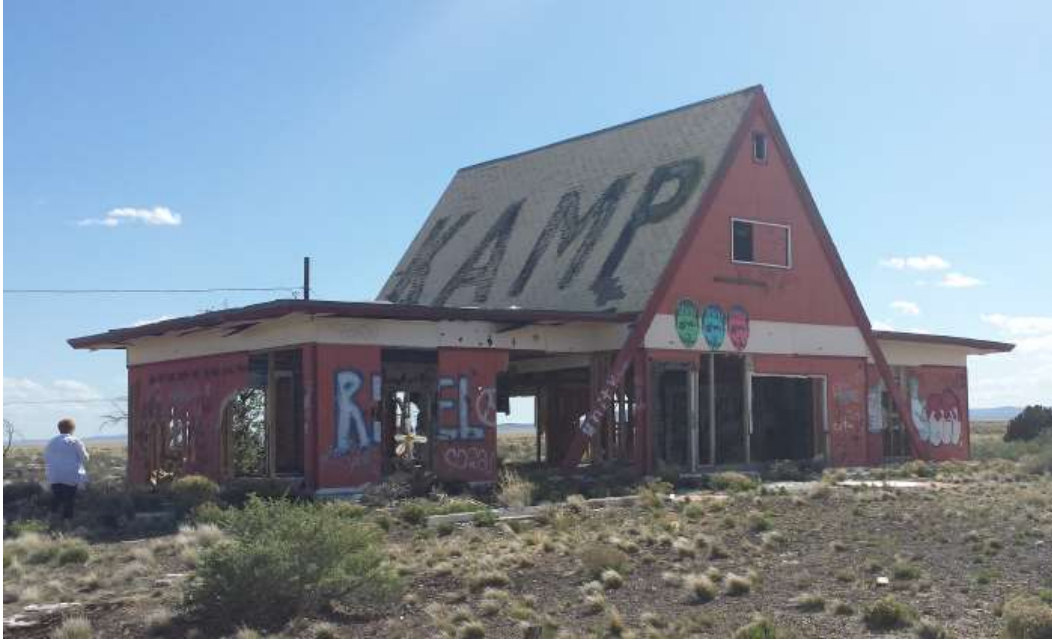
In 2015 the building was in a bad state and local (?) people were removing timbers to take away. In 2019 the destruction was almost complete:
